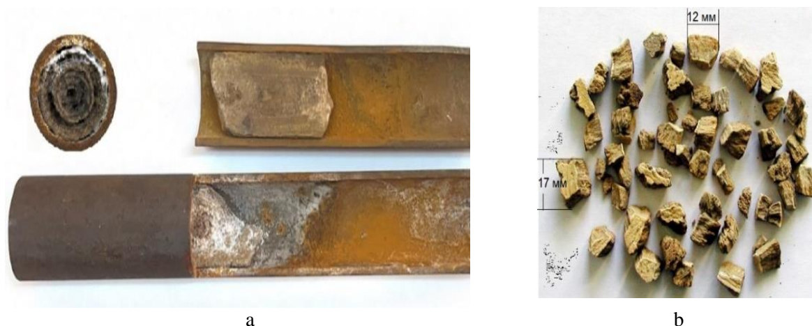
Figure 4. Samples of boiler pipes before and after cleaning using EHP — treatment: with hard deposits before processing; b) partially cleaned after processing, d = 51 mm
