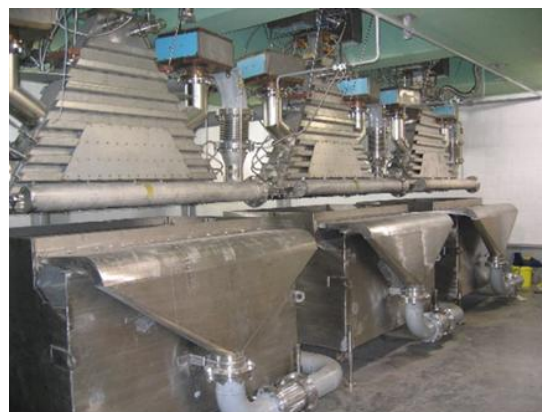
Figure 8. Waste water treatment room in the dyeing center. Daegu, South Korea
